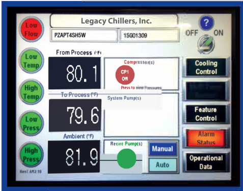
● Chiller Main Operating Screen
