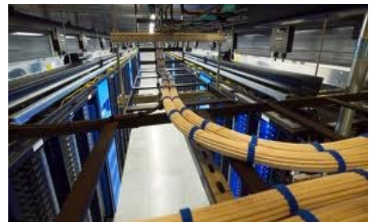
Legacy designed cooling and economizer systems for data and telecommunication centers
