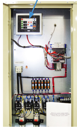
(Inside Mounted) Touchscreen Control Panel for Outside Chillers
